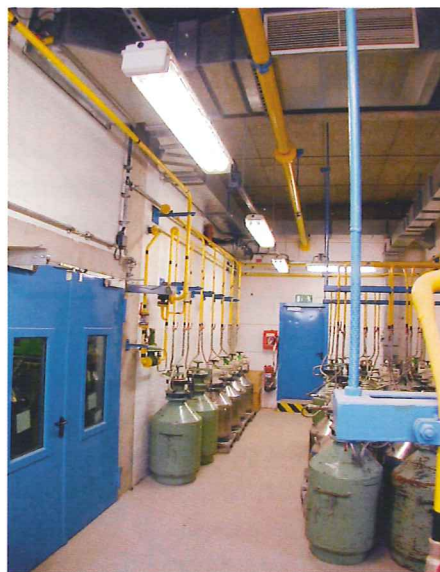
Figure 4: Approximately 120 light fittings from the R. STAHL works in Weimar ensure good and safe working conditions in both internal and external production areas. The fittings shown are EXLUX 6000 and 6008
