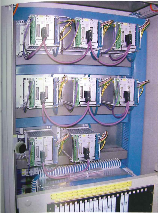
Figure 3: Switch cabinet in the control room with supply and signal isolating cards in 19" sub-rack. These cards enable intrinsically safe control of the local panels
